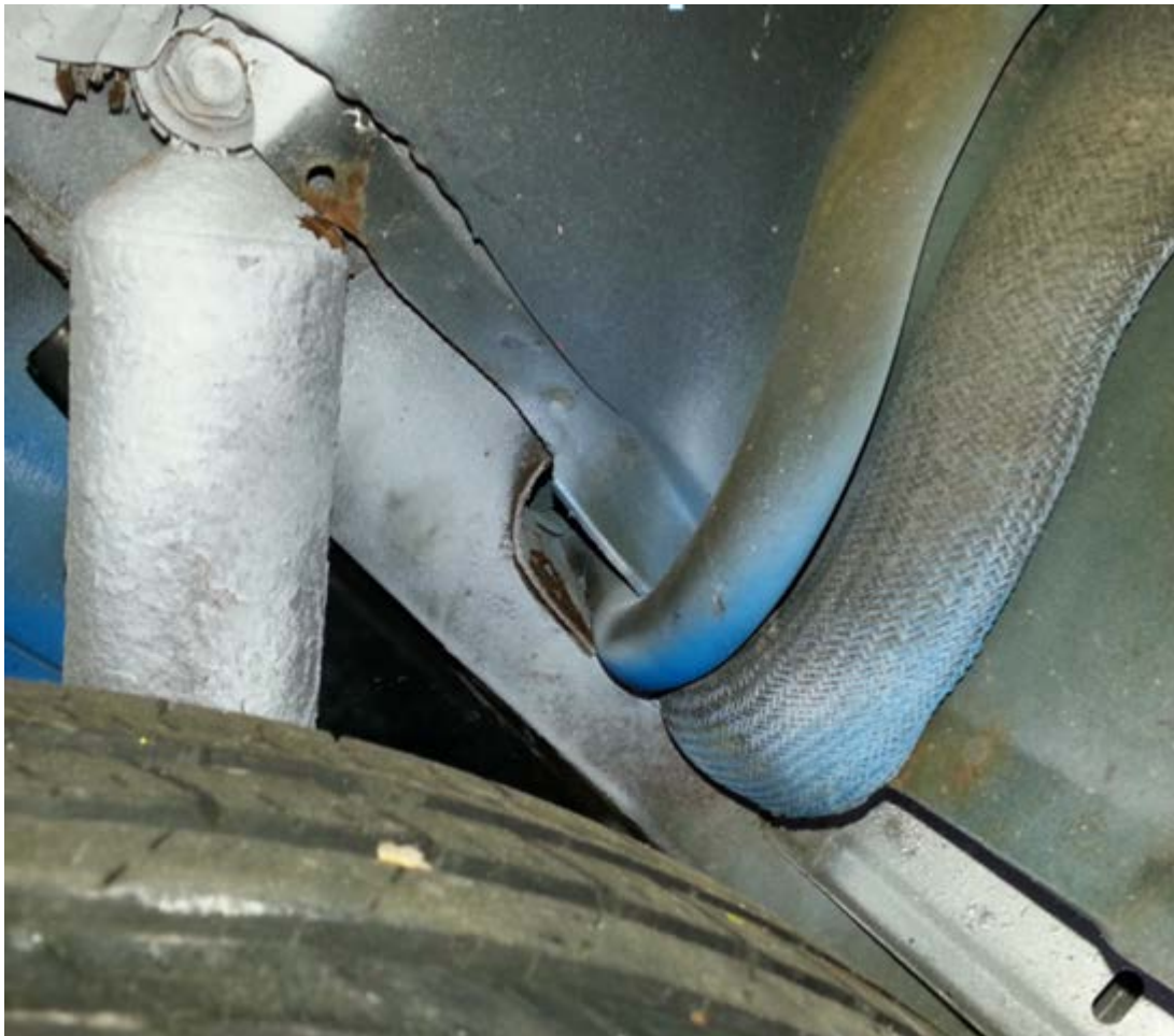
Figure 16 Test#7 Rail with rust reinforced by hitch-receiver bracket, hose not captured – moderately rusted vehicle
