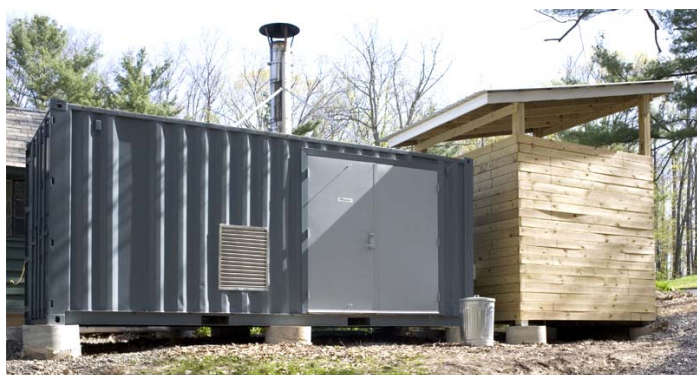
Figure 48 Cayuga Nature Center, in Ithaca, NY, has a 0.5 MMBtu wood chip-fired boiler (housed in a shipping container outdoors) that heats the main building, saving them about $15,000 each year on propane costs
