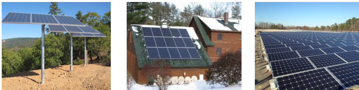
Figure 38 Ground-mounted system, Roof-mounted system and PV Farm
