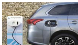
Level 2 (240V – Charging Station)
